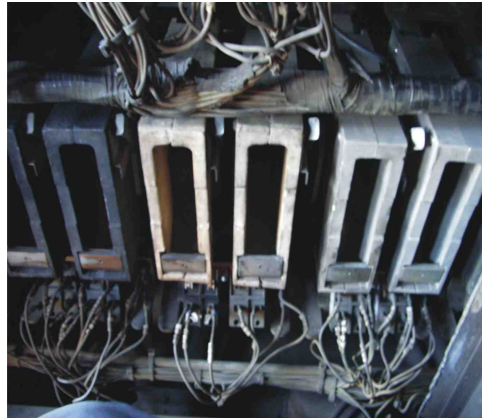
Engine room arc chute in an X class Locomotive. The black coloured arc chutes to the left were found to contain bonded asbestos.
