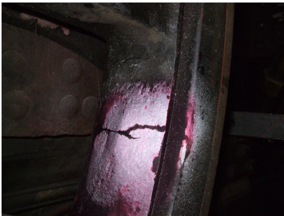
Figure 2 - Close-up view of one of the transverse fractures
