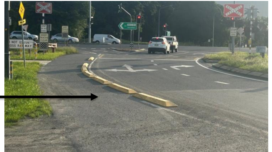
Semi-mountable curb barriers installed by road manager in 2026
